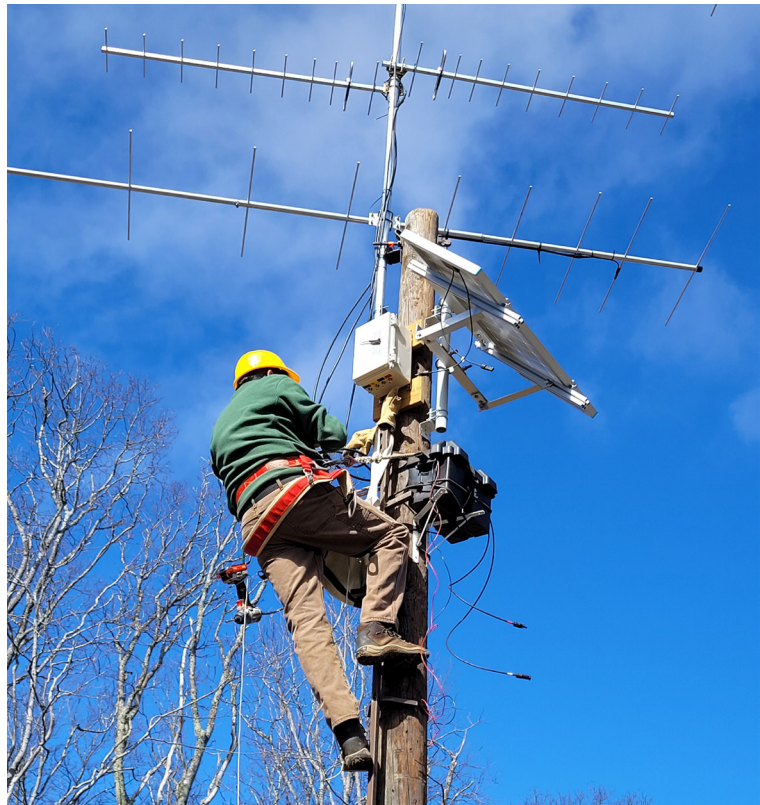
Kendrick Weeks connects the antennas to the receiver at WH Silver Game Land. The battery and charge controller are housed inside a battery box, mounted on a shelf bracket. The solar panel has its own mast. (Chris Kelly)
